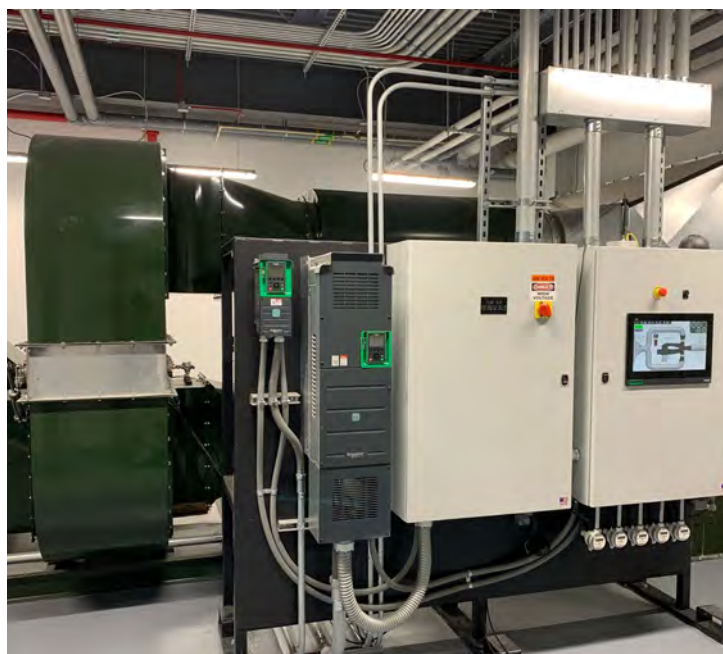
Fig 8. Typical air handling unit associated with forced air, ventilation and vacuum systems
