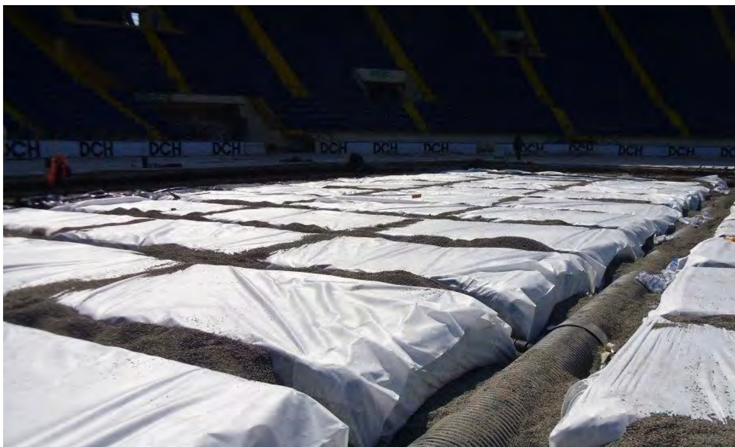
Fig 3. Drainage pipe in a lined trench
