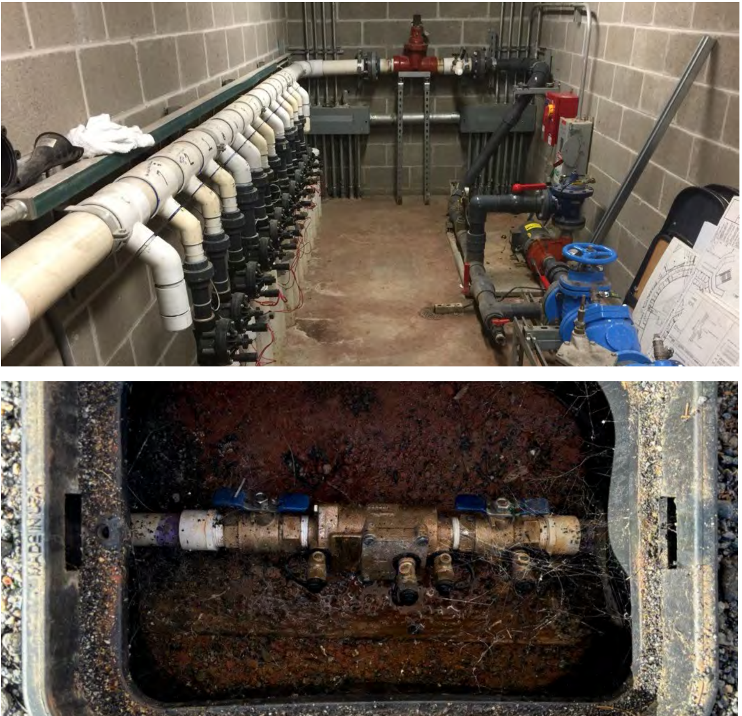
Fig 4. Aboveground irrigation valve room (top) and belowground irrigation valve box (bottom)
